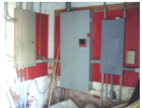
Figure II-91. Main electrical panels.
