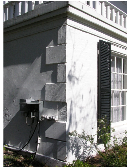
Figure II-7. Remnants of stucco quoining at the southeast corner of Orange Hall.
