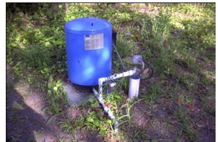
Figure II-99. Irrigation pump and pressure tank.
