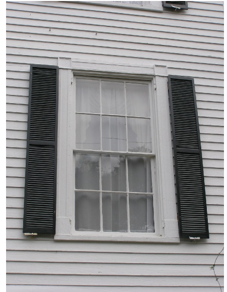
Figure II-14. Typical six-over-six, window located on First Floor, north elevation. Note replacement shutters are non-operational and narrower than original units.
