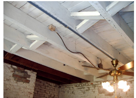
Figure II-93. Exposed wiring in basement.
