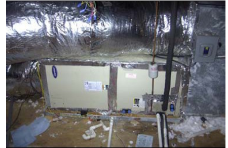
Figure II-82. Four ton fan coil unit in attic.
