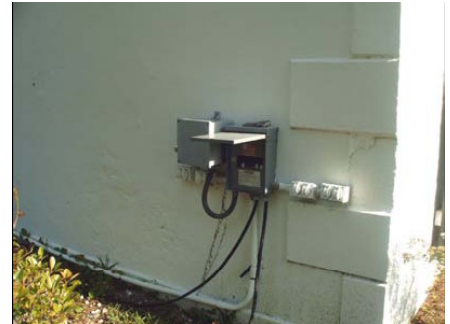
Figure II-95. Exterior power outlets.
