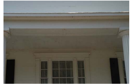
Figure II-32. Deflection of Lintel above Porch Columns.
