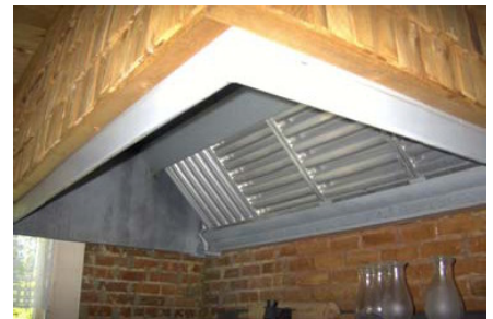
Figure II-87. Exhaust hood located in commercial kitchen.
