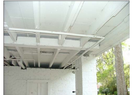
Figure II-29. Rear Porch Structure. Note 10" x 8" Girder is not connected to perimeter beam.
