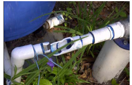
Figure II-101. Damaged irrigation water piping at pump.
