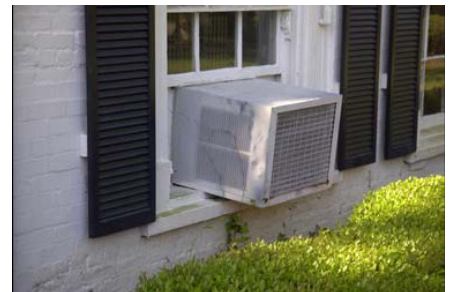
Figure II-86. Air conditioning window unit in basement.
