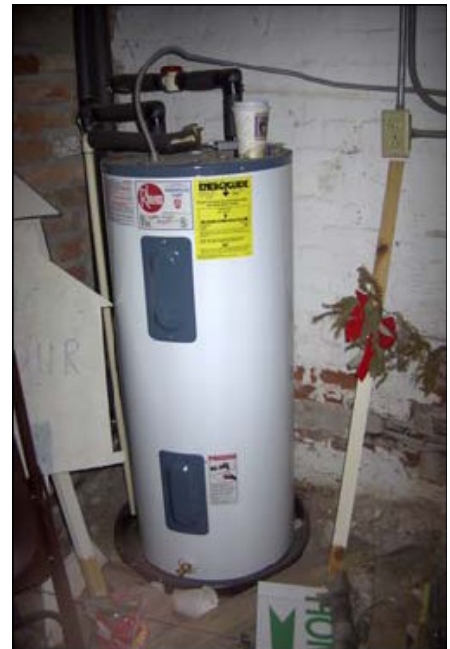
Figure II-97. Water heater in Electrical Room.
