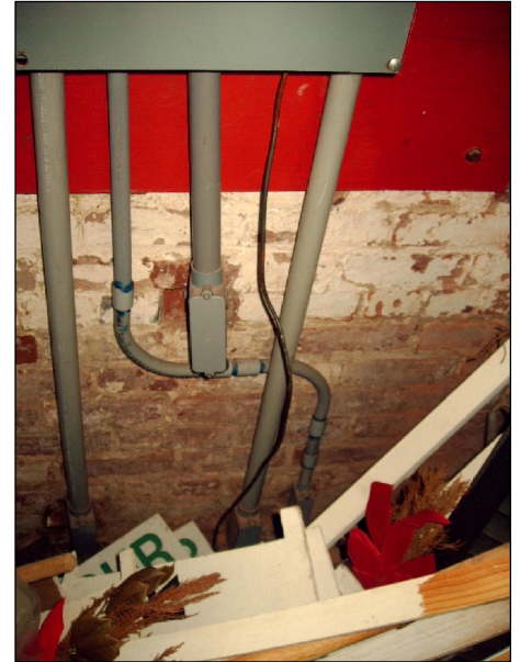
Figure II-92. Storage debris near electrical panel.
