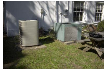
Figure II-83. Outdoor condensing units.
