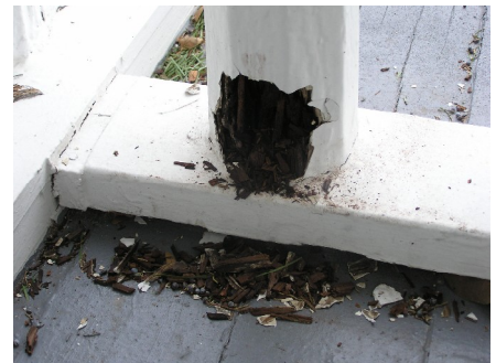
Figure II-12. Image showing deterioration of baluster at porch railina.
