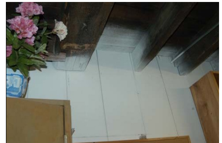
Figure II-27. First Floor Structural Members Severed at Stair.
