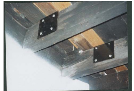
Figure II-30. Splitting of Ceiling Joists in Basement Level Hallway.
